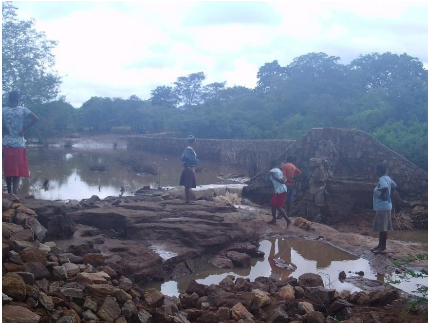
Figure 1. Nhora weir damaged earth wall in 2015
